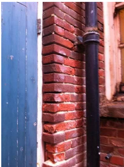
Eroded brickwork around pool fire exit
