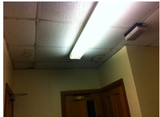
Water stained ceiling to first floor
