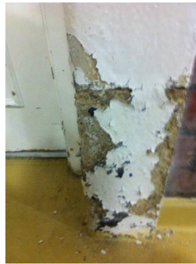
Deteriorated render to column in pool hall
