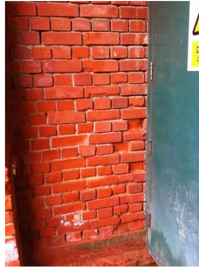
Eroded brickwork to basement
