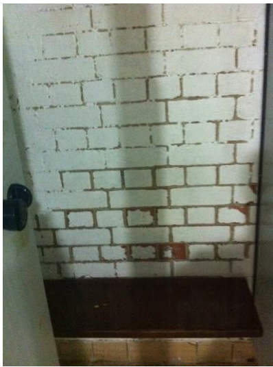
Eroded pointing to changing cubicles
