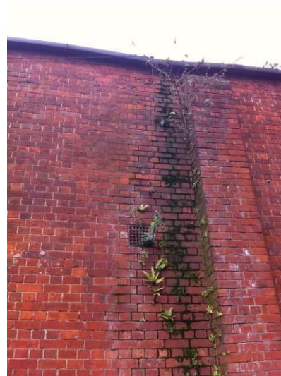
Leaking rainwater gutter
