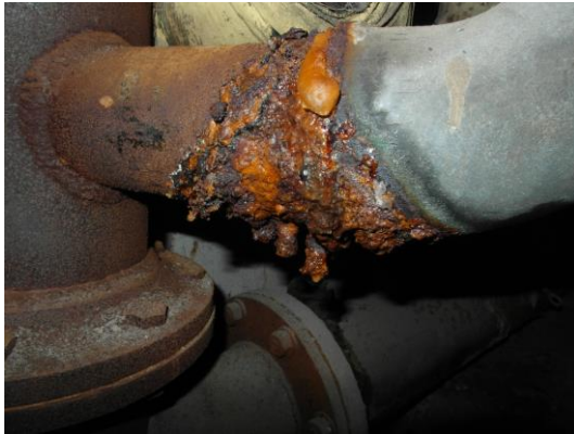
Corroded water pipe to pool
