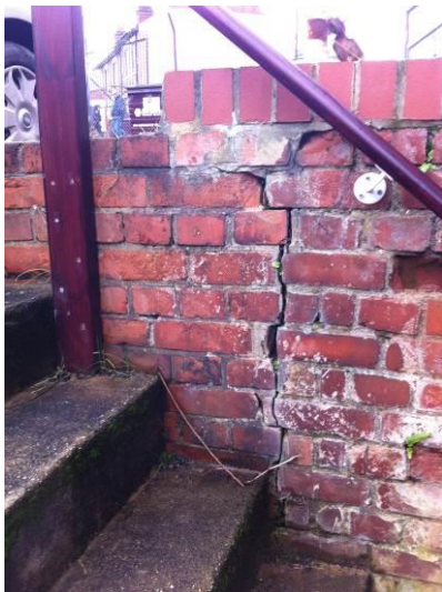
Crack to basement steps
